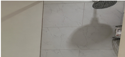
E-020 context Shower / tub area — tiles, grout, and fixtures Captured Jun 3, 2026, 11:37 a.m. Camera capture · EXIF b8c1d0e9f7a69230...
